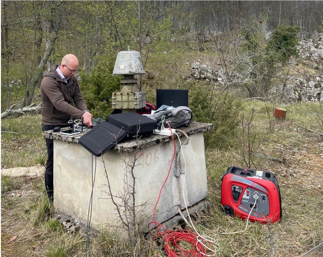
Figure 11 - RINICOM engineers setting up the mesh nodes in the field for creating communication infrastructure for transmitting IoT device data to the cloud
