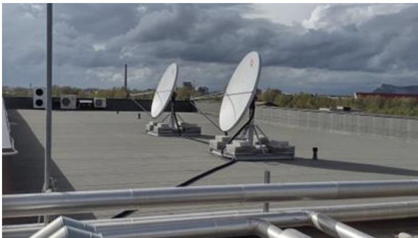
Figure 18 Satellite station installed at CMCC in Caserta.
