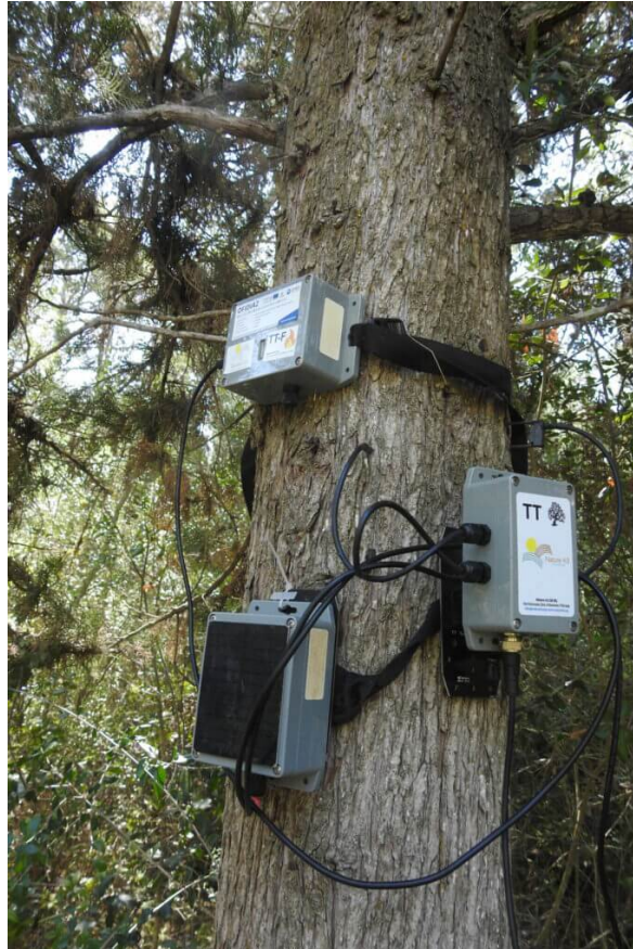
Figure 61 Example of an infrared fire detection system
