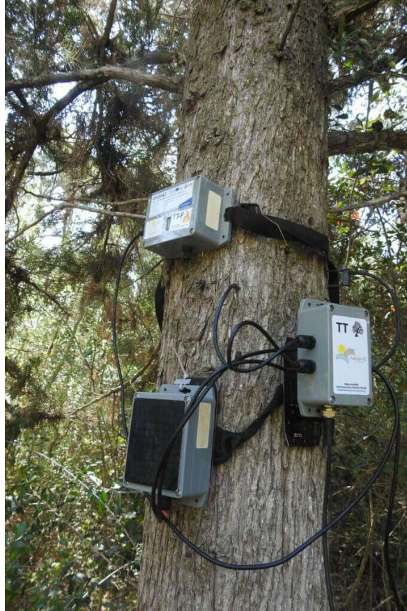
Figure 53 Example of an infrared fire detection system
